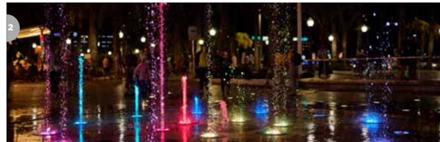
2 Installation of walkable fountains on the Paseo de la Explanada in Alicante.
